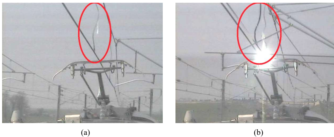
Figure 5.6: Dropper slacking: (a) Pantograph-catenary contact is maintained, (b) Loss of contact with arcing.
