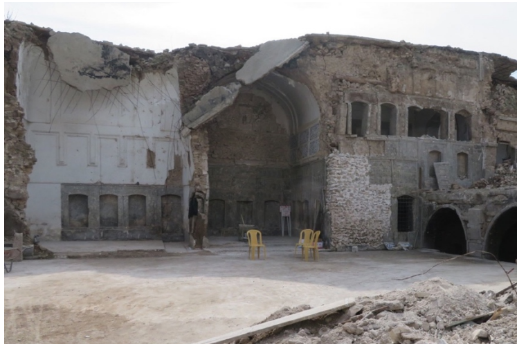
Figure 36. Al Tutunji house after destruction (Source: Iraq Heritage Stabilization Program).
