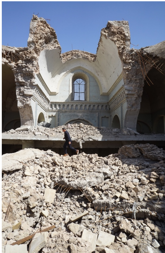
Figure 72. The interior of Al Tahera (Syrian-Orthodox) church located in the far north of the old city of Mosul, Bombed in 2017 (Source: UNESCO).
