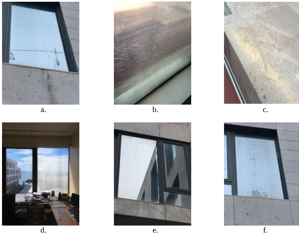
Figure 47. Examples of windows of the second case study building with the damaged SCF: a. tears; b. cracks; c. blistering; d. lack of transparency; e. detachment and; f. deterioration of the external layers of the film
